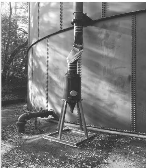
A new Dechlorinating Overflow Security Assembly (DOSA) installed at one of SJWC's water tanks
