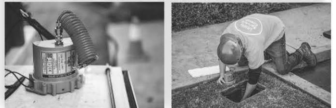
Newly installed tank mixing systems (top) and remote pressure monitors will provide continuous monitoring of SJWC's system and water quality
